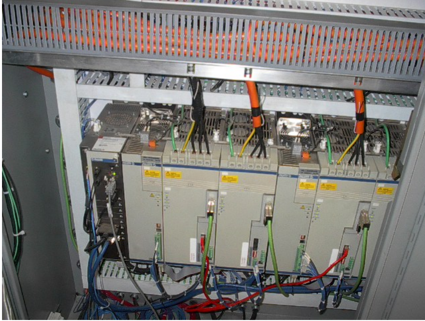
Inside Main Enclosure- lower left after install
