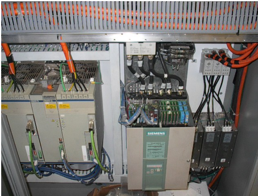
Inside Main Enclosure- lower right after install
